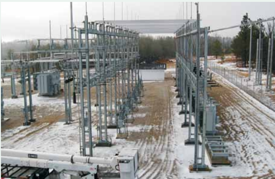
Doc's Road Substation went online in western Harnett County in early January 2010—just in time for the coldest weather.
